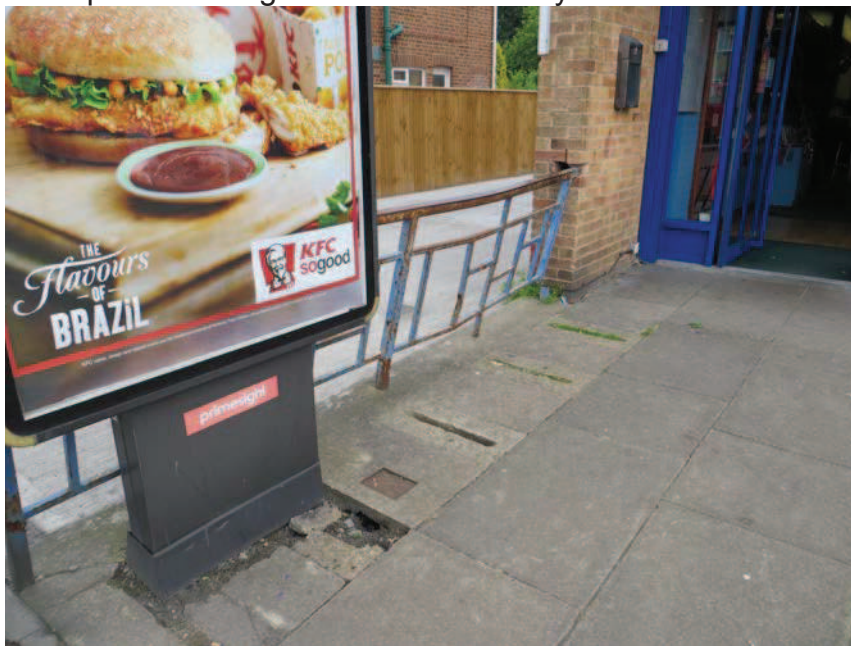
Example of Damage at Current Delivery Access
